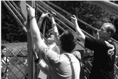
Construction of the yurt (left) in the international wilderness camp in National Park Bavarian Forest
